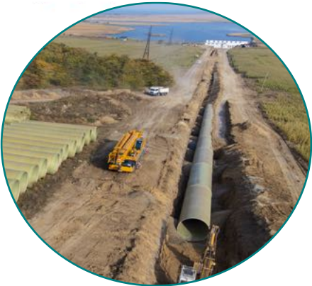
potable water mains and distribution networks
