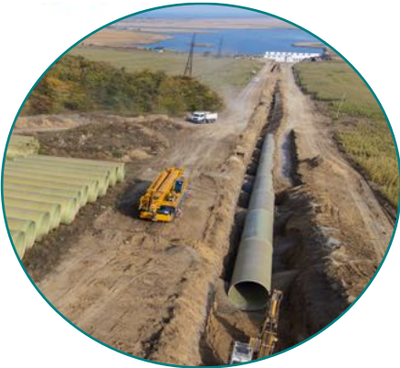
potable water mains and distribution networks
